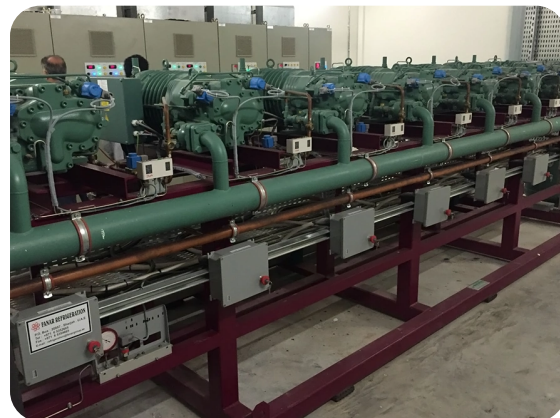
Industrial refrigeration plant - equipment must be evaluated at project operating conditions.
